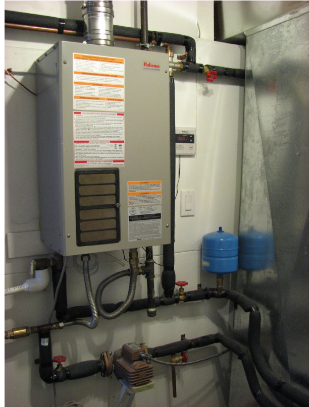
Figure 3. A picture of the installed test system. The system follows the schematic in Figure 2. The fan coil is on the other side of the cold air return. All hot water lines are insulated.
